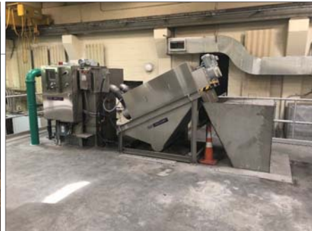
New PW Tech volute sludge thickener.
