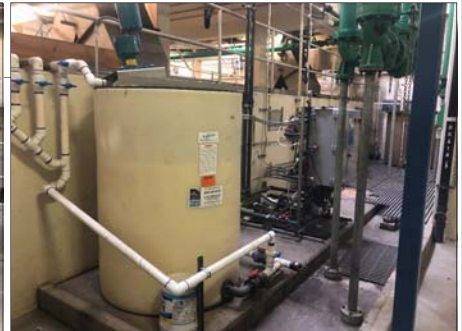
New polymer mixing equipment inside digester building.
