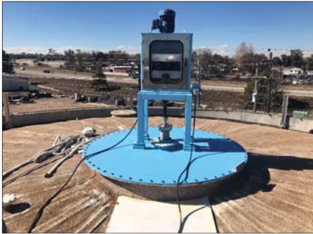
New Linear motion mixer on top of new anaerobic primary digester #3.
