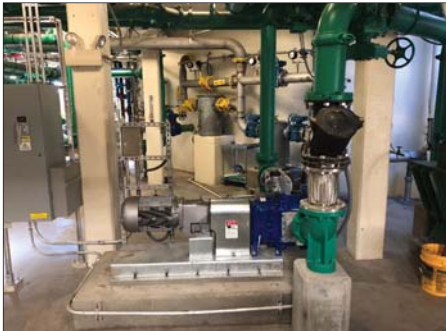
New sludge transfer pump inside digester building.
