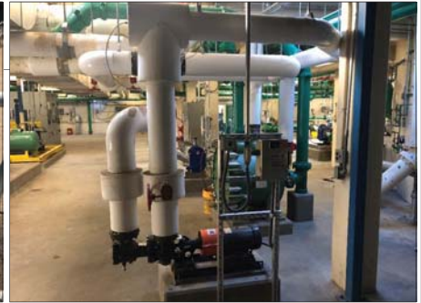
New sludge piping inside digester building.
